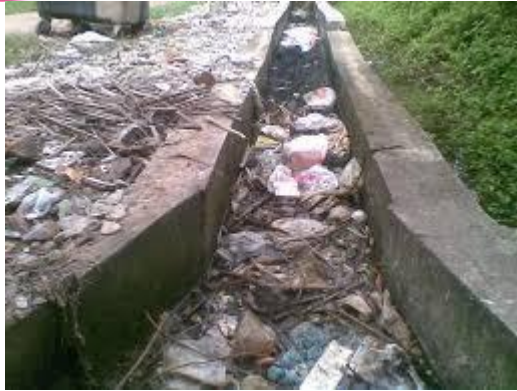
Fig 4 (a) Blocked Drains
